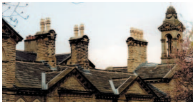
Chimney stacks and roof restorations are some of the works completed as part of a full programme of repairs funded by the City of Bradford Metropolitan District Council, English Heritage and the Heritage Lottery Fund.
